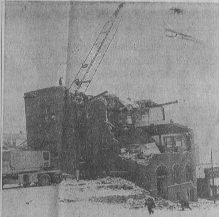
LANDMARK IS RAZED — Employees of Penn Ohio Demolition Co. on Friday began razing the old Altoona School of Commerce Building. This building also housed the second installation of the Bell Telephone exchange in Altoona. Wrecking crews will begin razing the Levan house on Wednesday or Thursday of next week.
